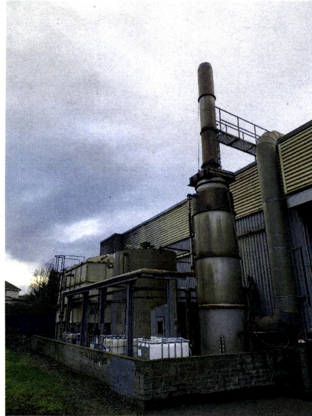
Figure 1: Alert Packaging abatement system enclosed with concrete bund wall
